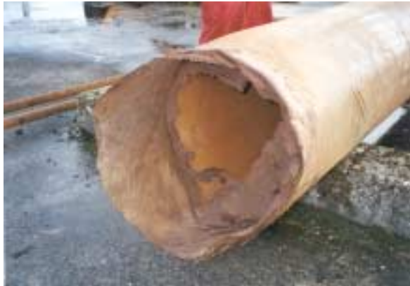
Fig. 4-5: Point of fracture of FRP string
