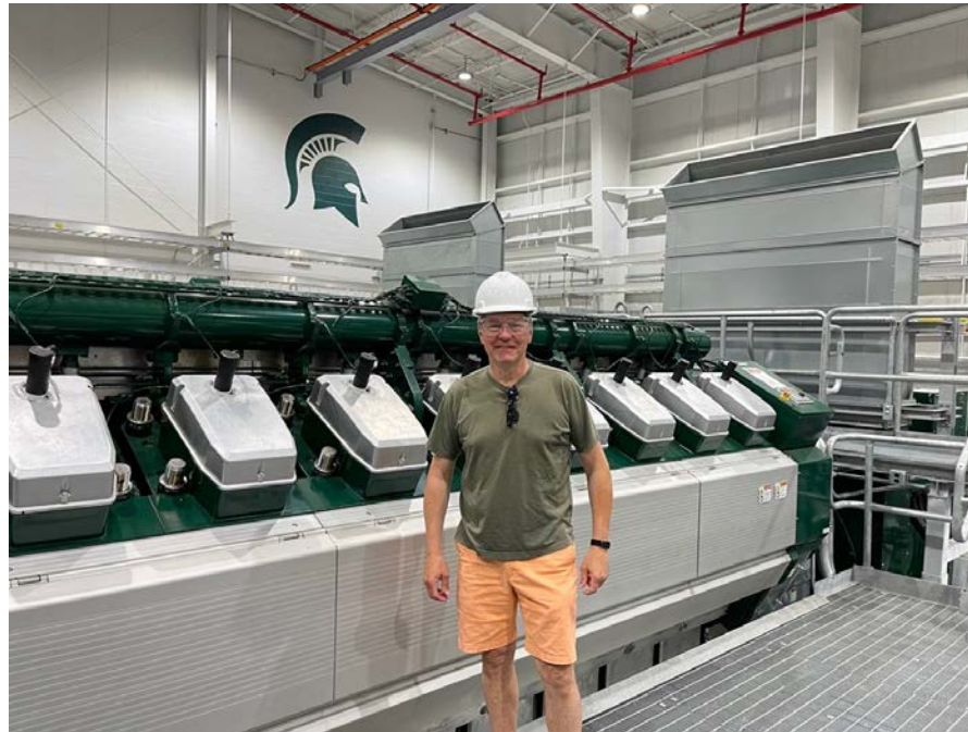
MSU's new 30 MW RICE plant: need 13000 of these
