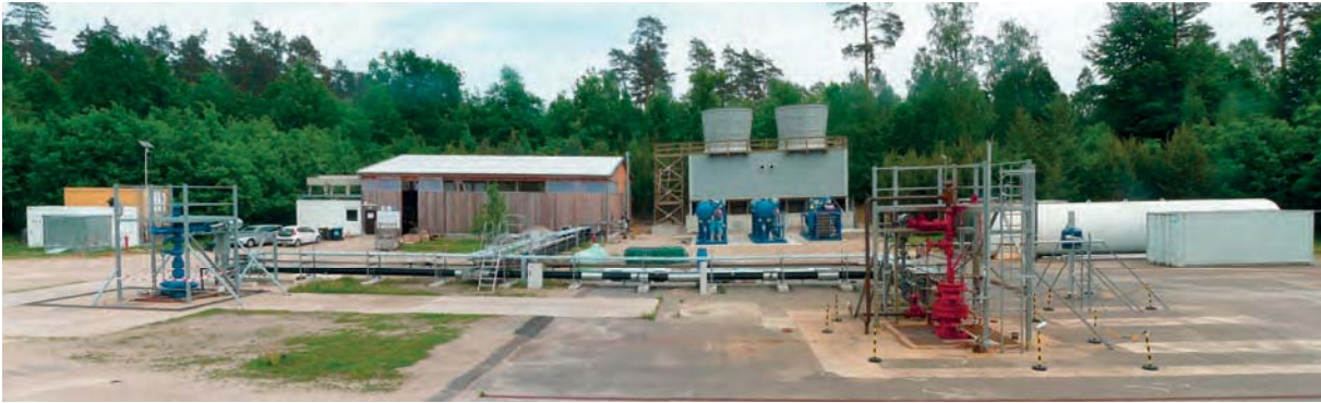
Fig. 5: Surface installations at the geothermal research platform Groß Schönebeck with production well (red), injection well (blue), function hall (rear left) and ORC-plant with cooling towers (rear right).
