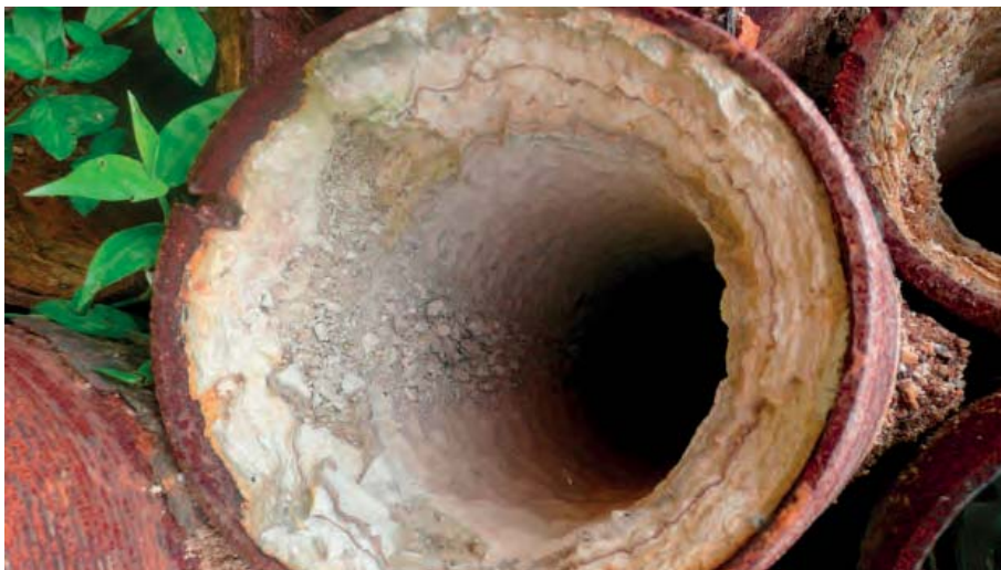
Fig. 17: Plant components at an Indonesian geothermal power plant showing massive silica precipitation (scaling) and a significantly reduced cross-sectional area available for flow.
